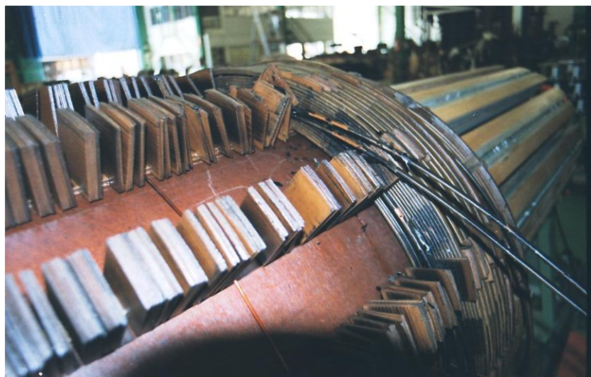
FIG 1. Breakdown of the dielectric system in a power transformer column. Courtesy from Electric Works Molina, Córdoba.
