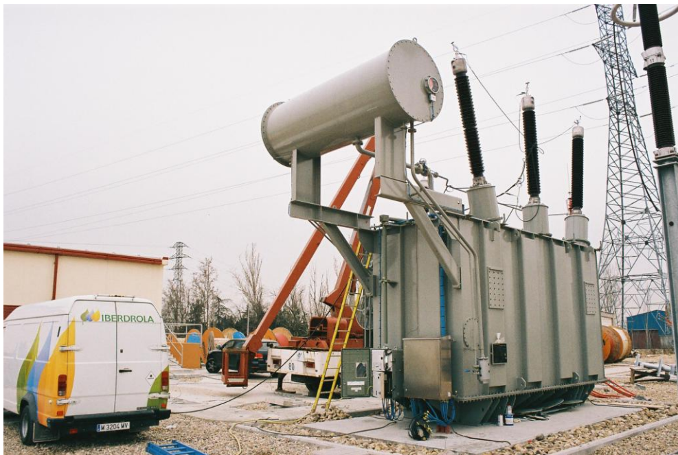
FIG 2. Field testing of a power transformer before putting into service (50MVA).
