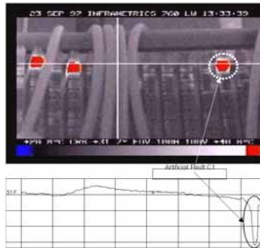
Fig. 5. Correlation of a Full flux test to reduced flux test (EL-CID). The plot below is the indication of the upper fault.
