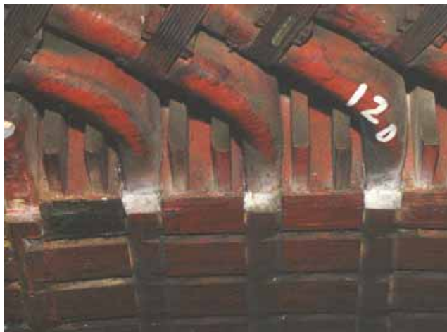
Fig. 3. Dust associated to partial discharge in endwindings.
